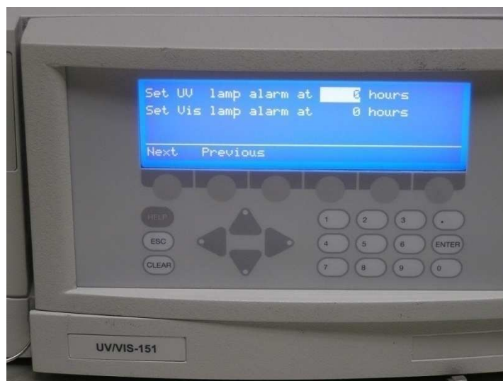
Figure 5-6 UV Lamp Alarms
